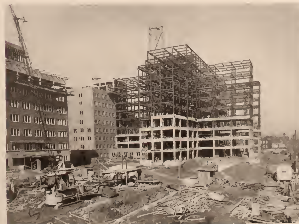
Advances in design and construction of highways, bridges, hospitals, and public buildings are credited to engineers in the career civil service. The modern hospital pictured under construction is one of a number of major construction projects designed by Federal engineers.
